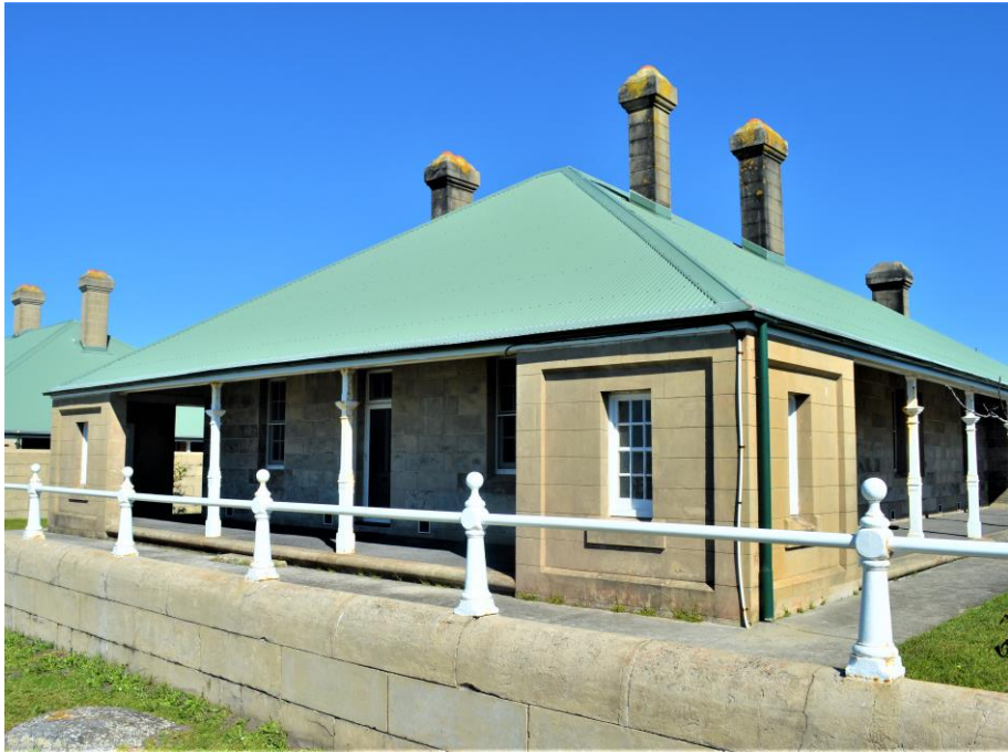
One of the lighthouse keeper's cottages, constructed of solid, pre-cast concrete blocks.
